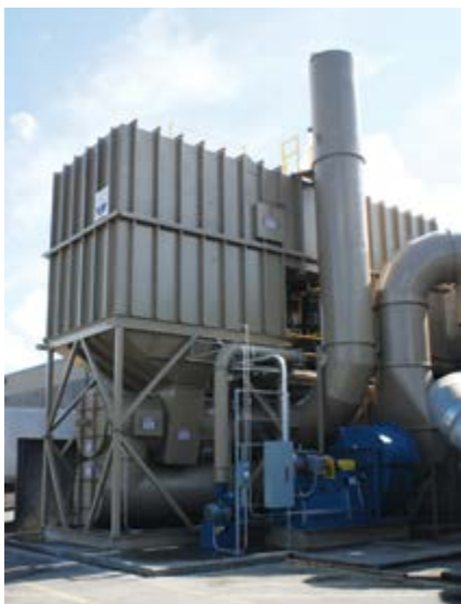
Example of a 50,000 SCFM Regenerative Thermal Oxidiser (RTO) for the printing industry
