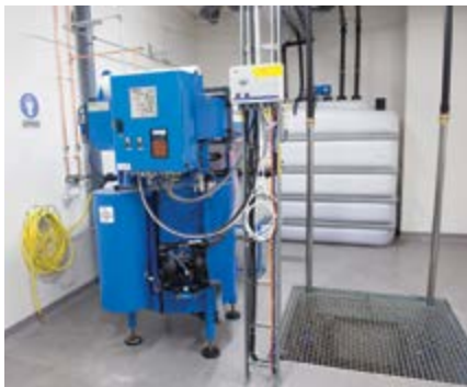
Hot Screen has its own internal waste water treatment plant
