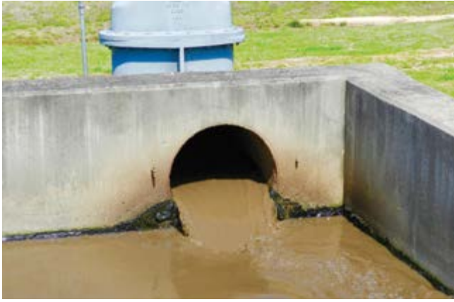
Raw sewage enters the treat-plant into the oxidation ditch
