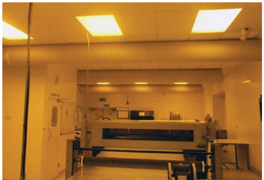
This picture shows air socks to diffuse the air flow from the HEPA filtered air conditioning
