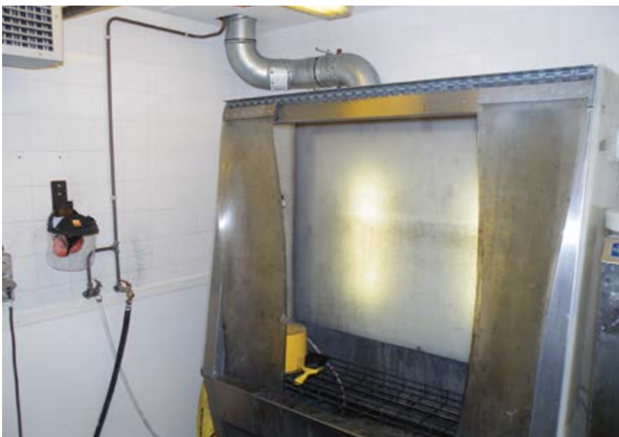
Cleaning booth with good ventilation
