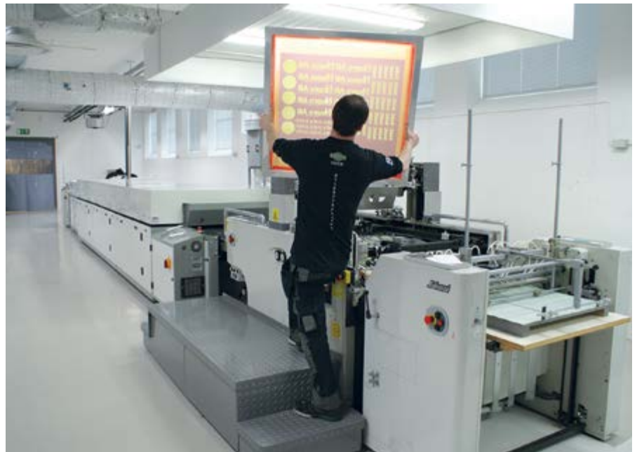
A recent Natgraph installation resulting from testing at the company's Drying Solutions Centre
