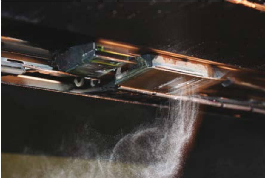
This picture shows abnormal jet over-spraying in action
