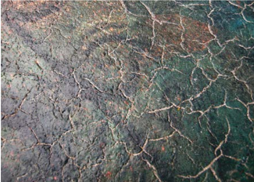
Figure 2: Close-up of the cracking and micro-fracturing of the product, allowing water to drain through or run off the graphics easily
