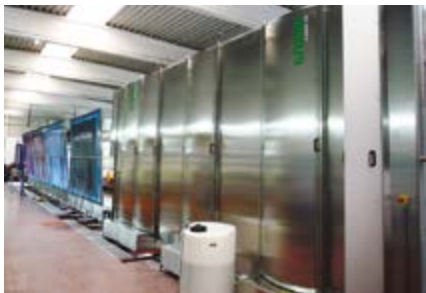
An automatic in-line washing installation
