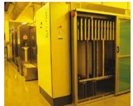
The In-Line screen cleaning plant with de-stacking and final drying
