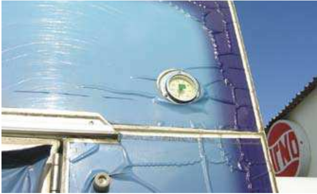
When the protective film and the printing substrate are not 'like with like' products, tunnelling and delaminating usually appear
